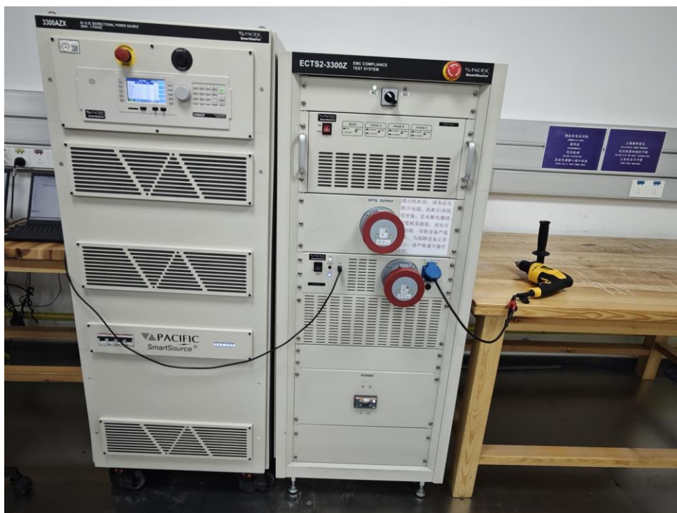
Photograph 6: Set-up for Harmonics, Voltage Fluctuation and flicker
